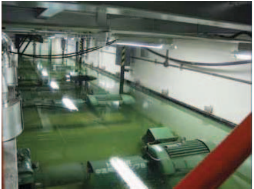
Figure :7 Flooded Emergency Generators Located in the Basement of Turbine Building Unit 3
